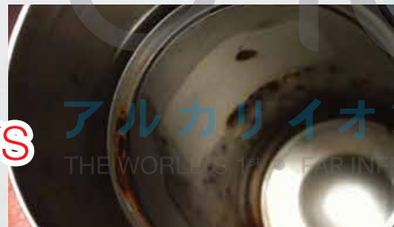
Metal water tank Releasing heavy metals
